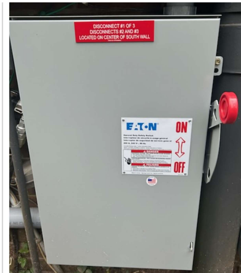
Example of correct labeling on disconnect.
