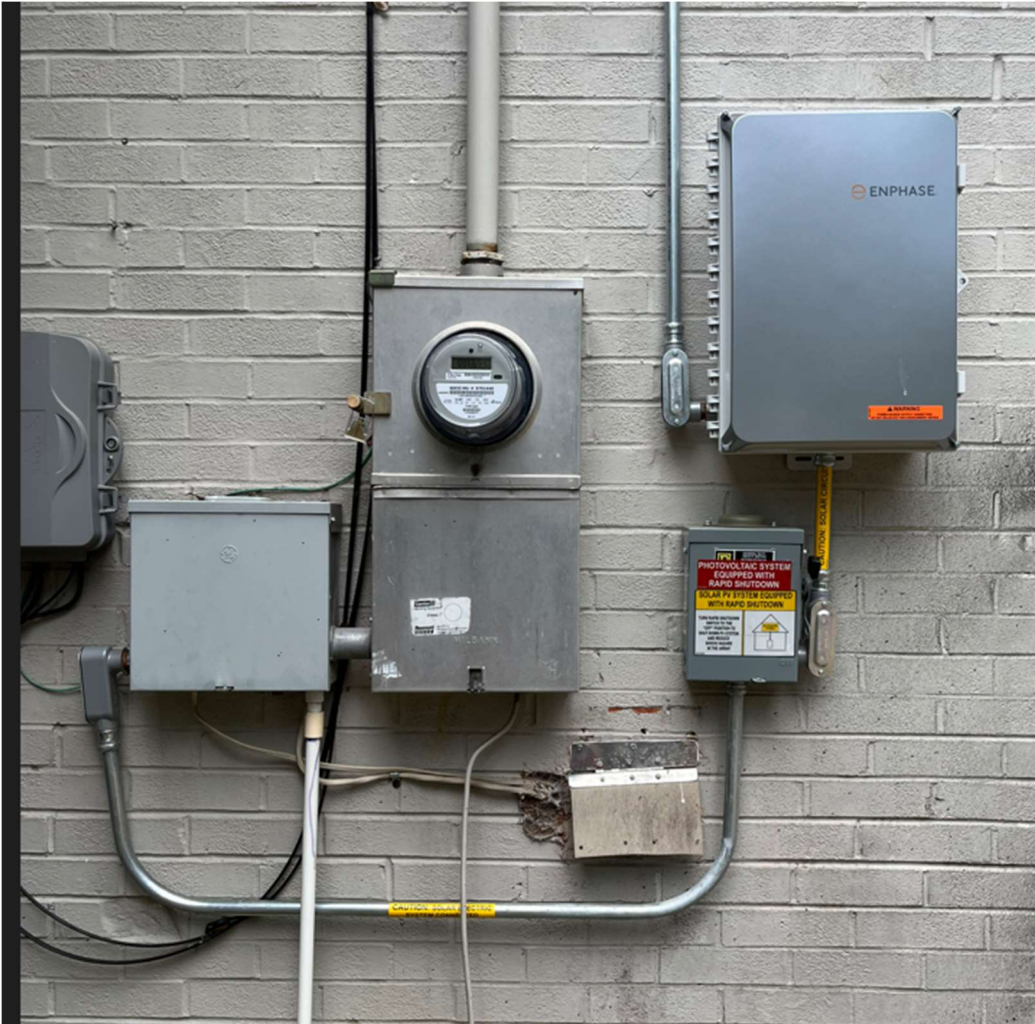
Example 2: Post installation picture of meter socket and newly installed PV AC disconnect
