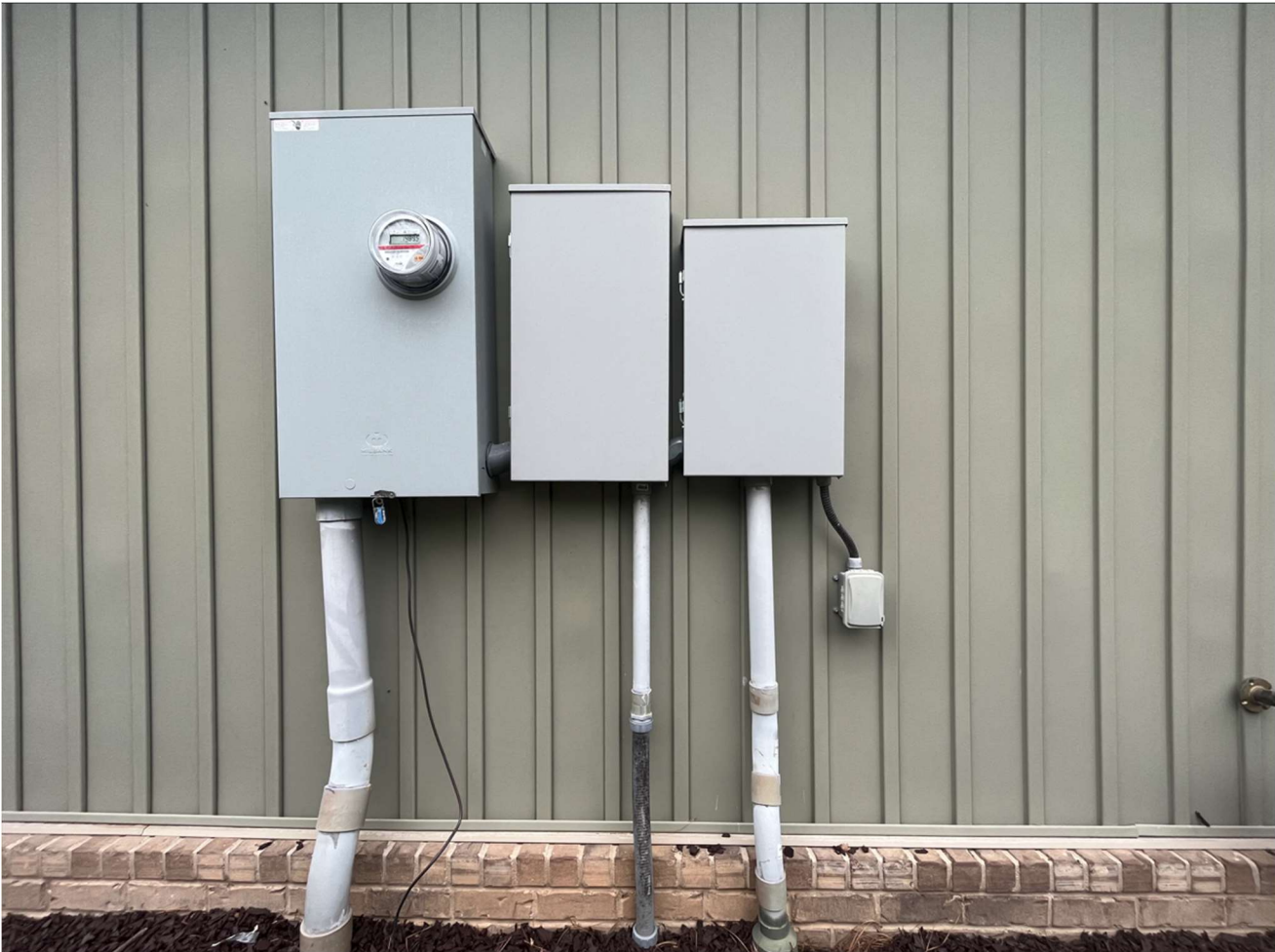
Example 1: Pre installation picture of existing meter and main service panel
